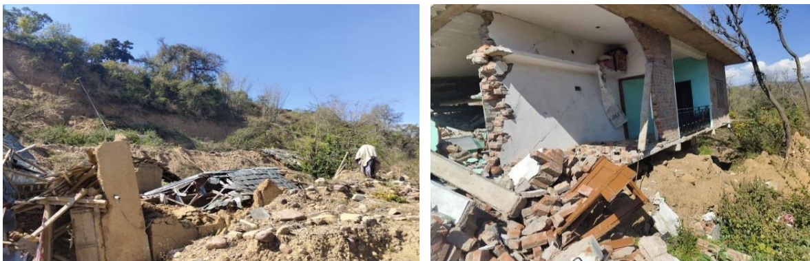
Fig 4 Collapsed houses and cowsheds
